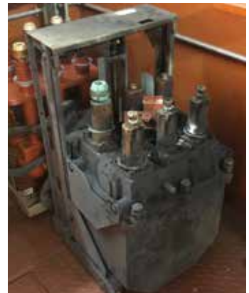
Overheated SF6 Breaker
